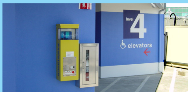
Custom-painted CB 2-e wall mount unit in one of Yahoo!’s parking garage provides high visibility. At a touch of a button, an employee or patron is able to immediately communicate with security personnel. The blue strobe notifies security of the person’s exact location.
