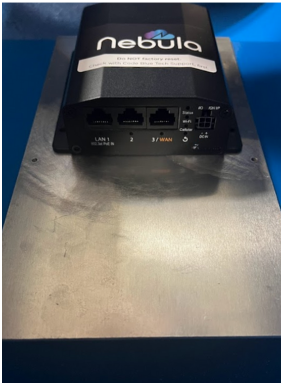
Router & Hanger Plate Installed on Communication Plate
