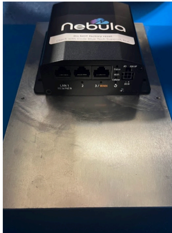
Router & Hanger Plate Installed on Communication Plate
